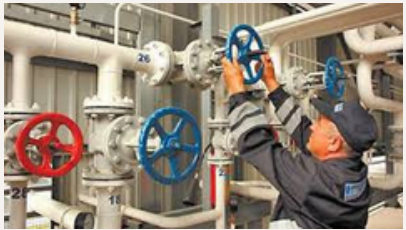
Municipal enterprise Stryiteploenergo Source: Stryiteploenergo
